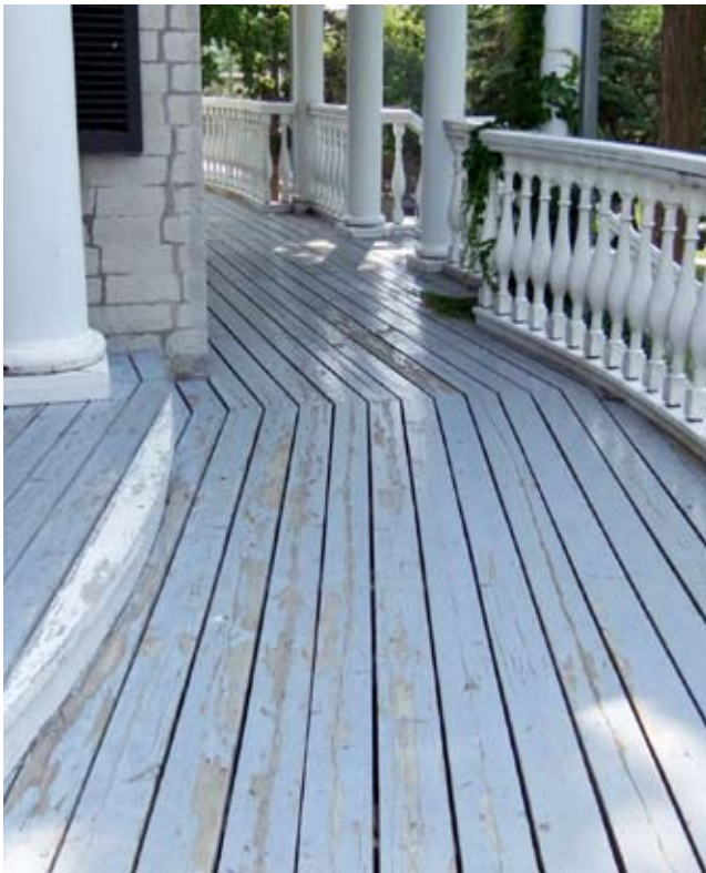
Paint failure on wooden veranda
