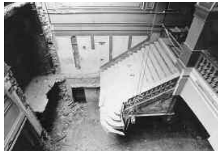
The Elgin and Winter Garden Theatre Centre (Toronto). In 1987, a basement is excavated under the lobby corridor, and the grand staircase is suspended in the air.
