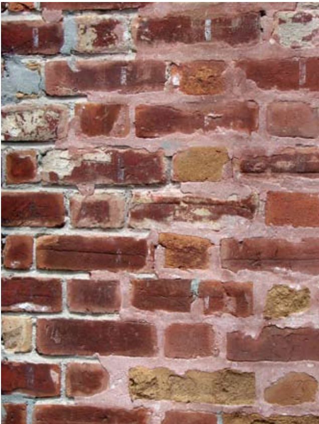
Inappropriate repointing has damaged these masonry units. The harder, cement-based mortar has caused the bricks to spall. The mortar has also been carelessly applied, thereby compromising the architectural character of the building.
