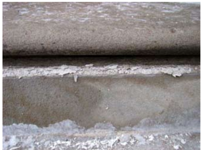
These steps were repointed during the onset of cold weather. The mortar was not able to achieve its intended structural strength because of the temperature. Consequently, the mortar prematurely failed during the same winter season.
