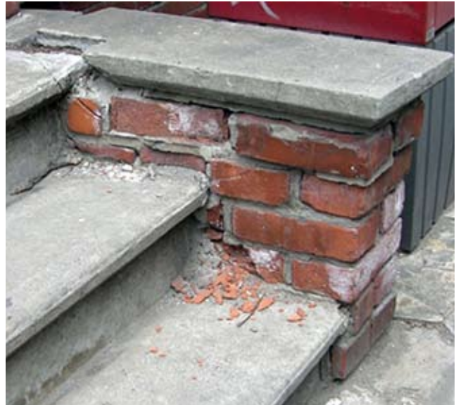
These bricks were repointed with a cement-based mortar. The high, compressive strength of the mortar, compared to the masonry units, has caused the bricks to spall, leading to irreparable damage.
