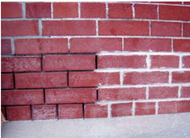
This mock-up reveals that the cutting-out methods employed by the contractor widened the joints and damaged the brick. The mortar mix does not match the original pointing in composition, colour or profile and the mortar itself was inappropriately applied.
